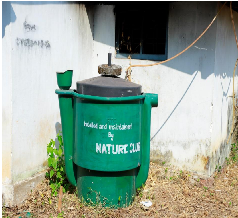
Bio Gas Plant
