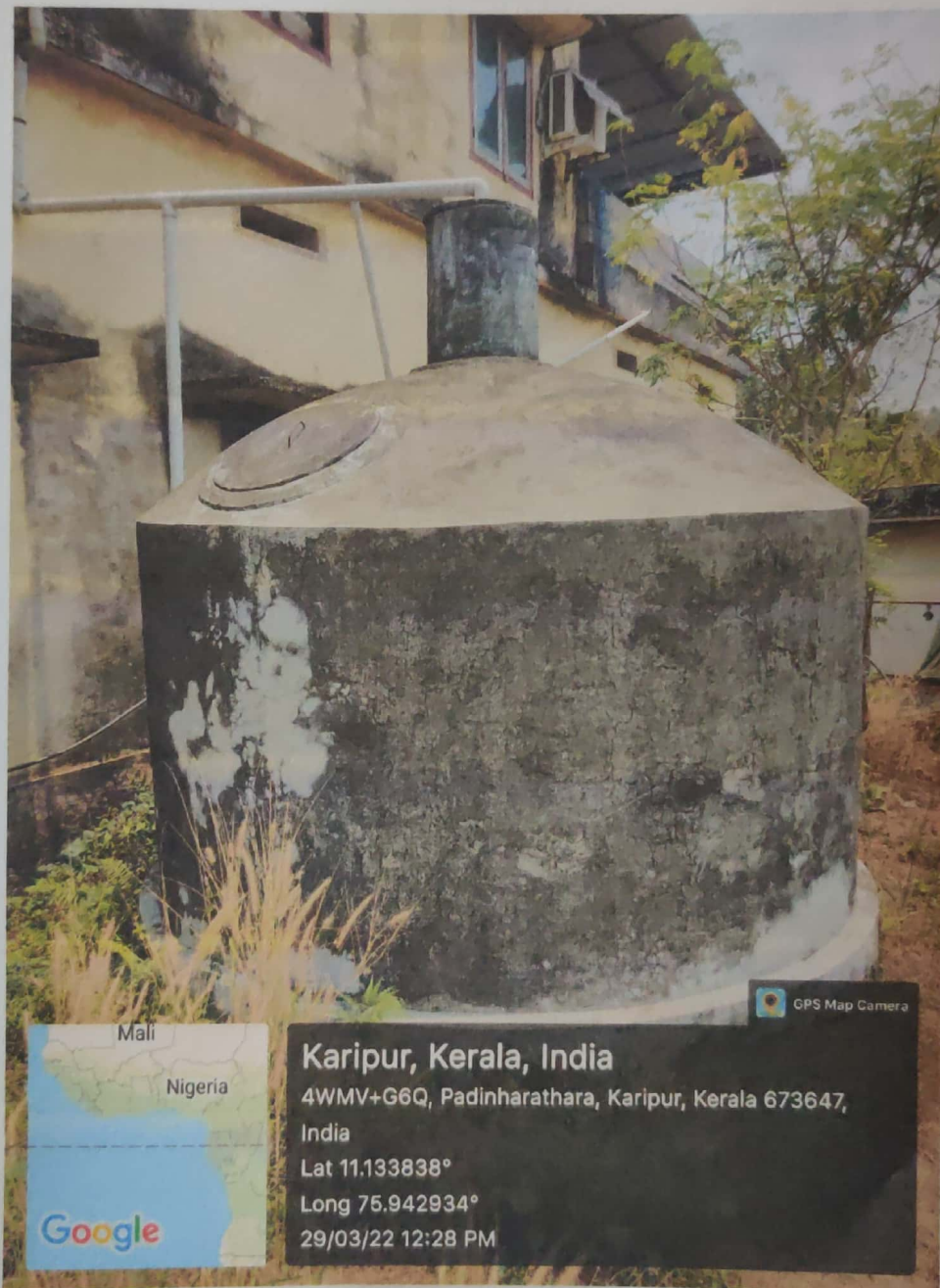
Rain water harvesting Tank
